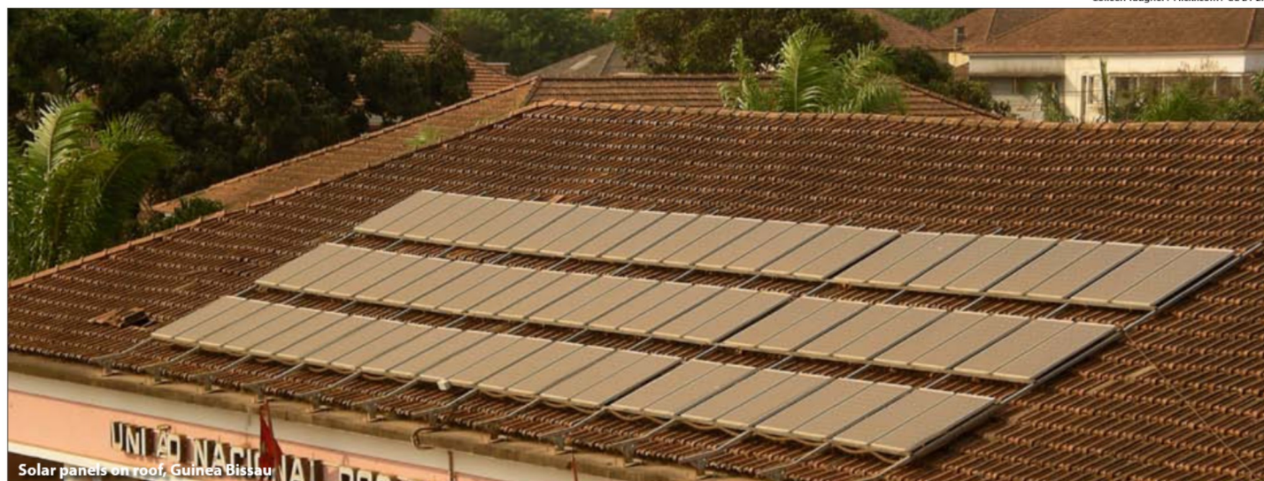
Solar panels on roof, Guinea Bissau
