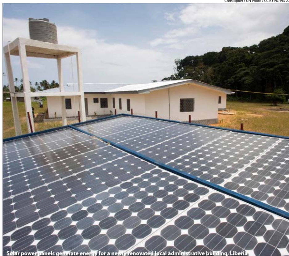
Solar power panels generate energy for a newly renovated local administrative building, Liberia
